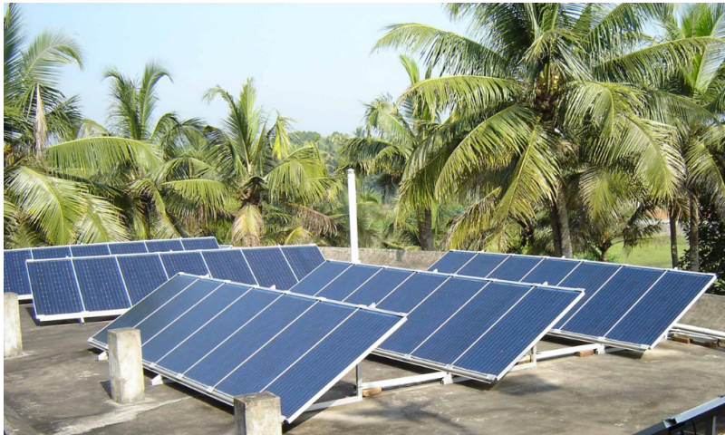
5 Kw Solar Power Plant Installed in Mithradham (1999)
